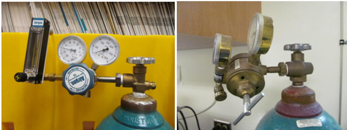
Figures 1 and 2: Gas cylinders with inappropriate use of Teflon tape.
