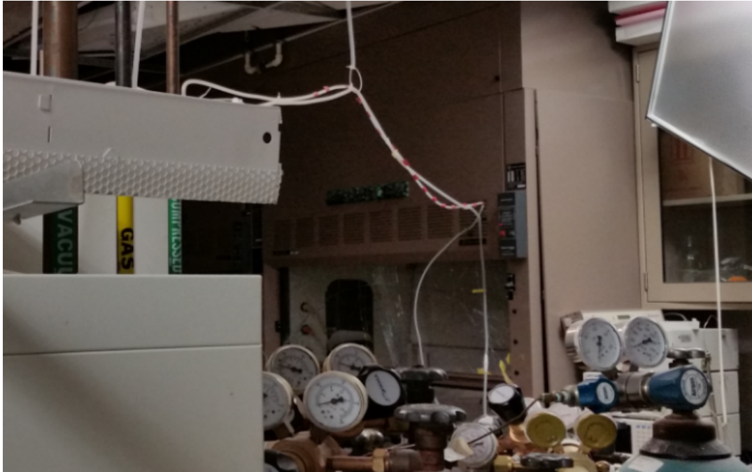
Figure 5: Polyethylene tubing hung from the drop ceiling and only marked with colored tape.
