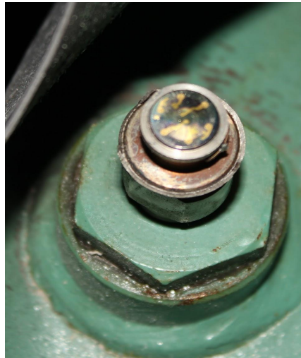
Figure 26: Pressure gauge diaphragm still attached to the threaded gauge stem that was still threaded into a bushing on the tank. On the external surface (non-wetted side) of the diaphragm one can see markings where the strain sensors were attached to the diaphragm.
