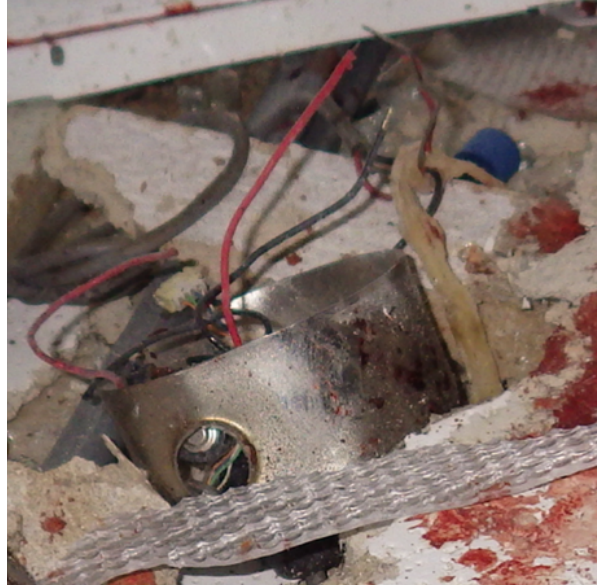
Figure 27: Pressure gauge housing as found by HFD
