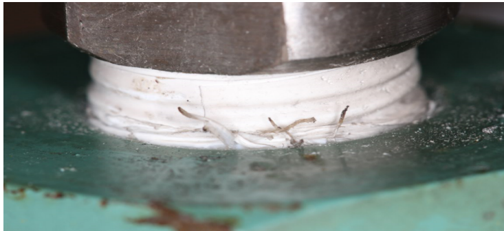
Figure 32: Photo of gauge stem Teflon tape that appears to be charred and melted.
